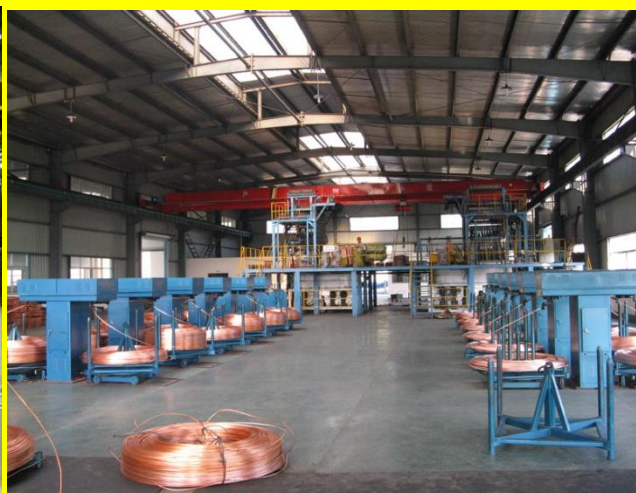
Attachment No.7 Horizontal Strip Casting Line
